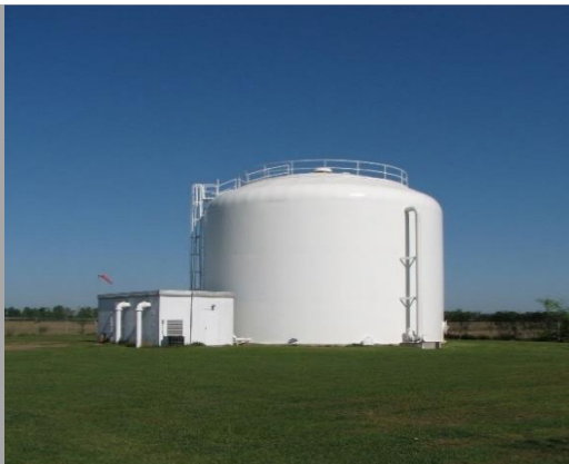
Water Plant #4 (Wilson Plant)
