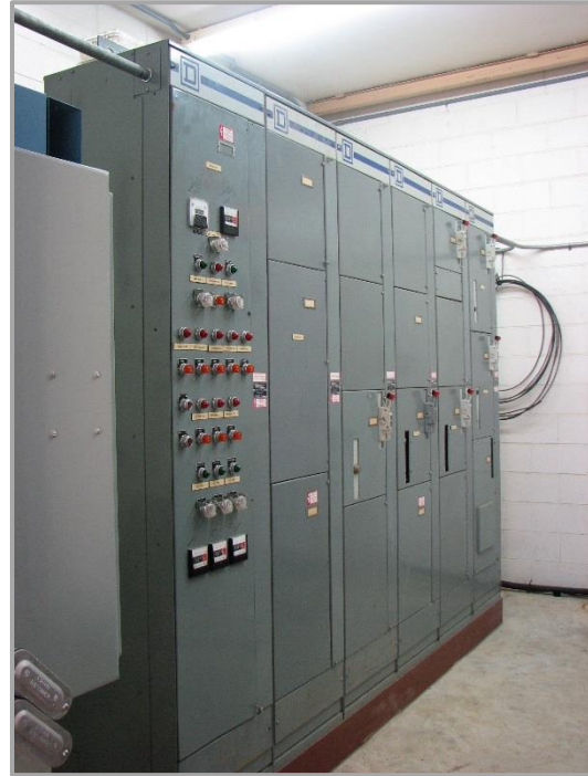
MCC Panel at Water Plant #1 (Monseratte Plant)
